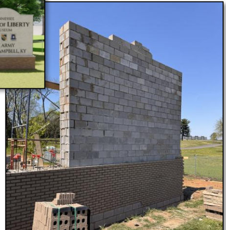
The public entrance wall and signage under construction the intersection of Tiny Road and HWY 41A
